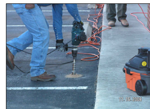
Figure 3. Drilling of holes to place soil gas collector tubes near the Savings Square Shopping Center. (Source: EPA)
