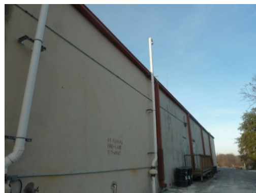
Piping used to discharge vapor collected from underneath Building 1 as part of the soil vapor mitigation system at Savings Square Shopping Center.
