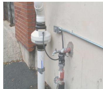
Figure 4. Example of vapor mitigation system recently installed at the Savings Square Shopping Center.
