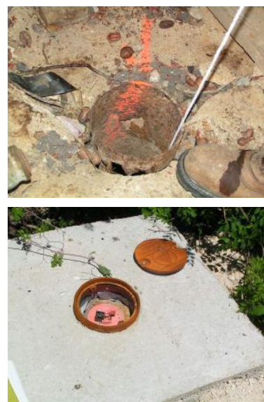
Figure 4. The top photograph is a well with corroded surface casing and broken concrete slab. The bottom photograph is of a secured well with a new surface completion (i.e., concrete slab) and locking well cap.
